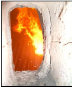
Fig. 7. Flame condition at initial oil firing
