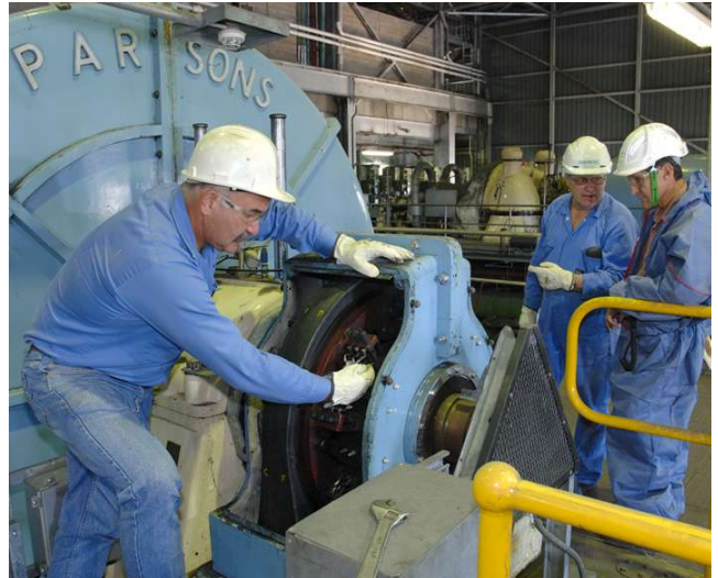
CS Energy's Dr Chris Spero (right) discusses the condition of the unit 4 generator at Callide A with a Siemens crew.
