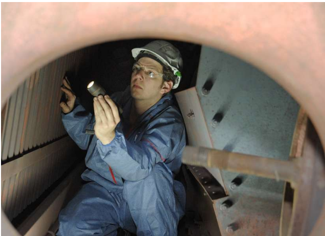
CS Energy project engineer Franco Montagner inspects the Callide A boiler, which will be retrofitted with oxy-firing technology.
