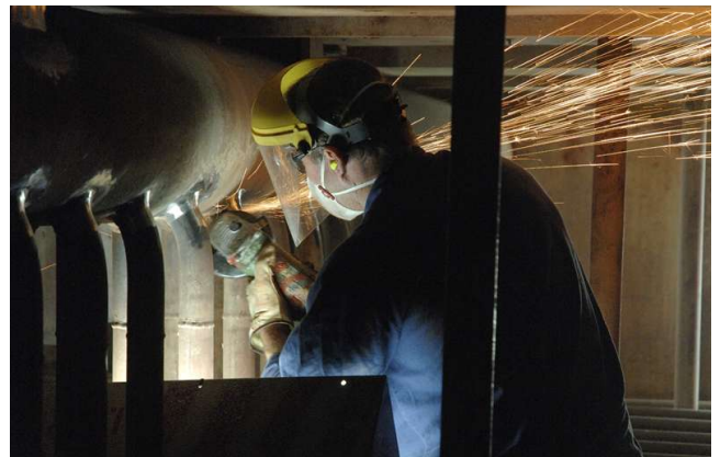
The Callide A condition assessment included checks of the integrity of welds in the boiler. Grinding preparation work was the first step in this process.
